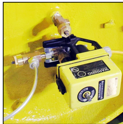
IV-810 with emergency shutoff actuator on a ton container with flexible connector.
